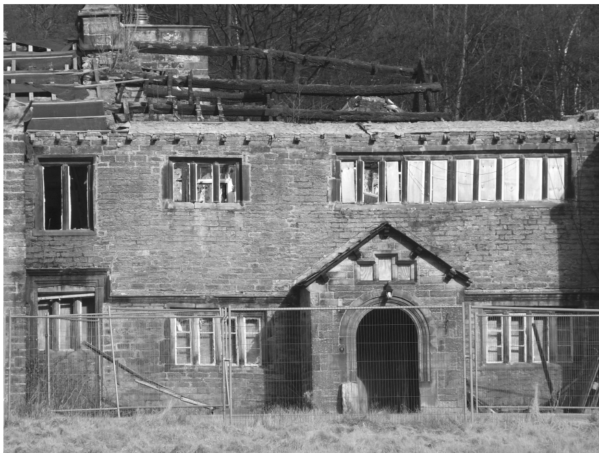
The Holme with its fire damaged roof and derelict main entrance in 2009
